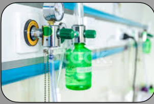
HOSPITAL OXYGEN SYSTEM
